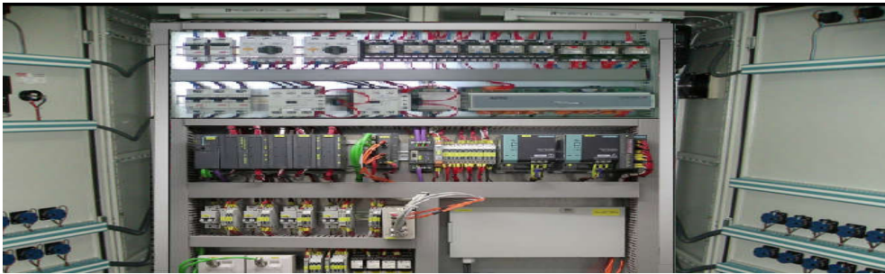
Figure 3. Created power transformer measurement panel
